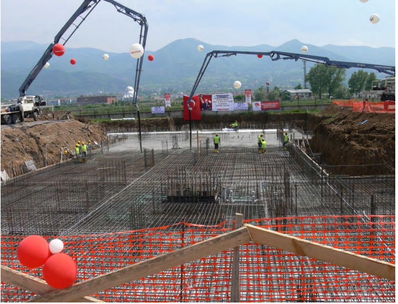
SAĞLIK MESLEK LİSESİ İNŞAATI (ANAHTAR TESLİM)NURSERY AND HEALTH HIGH SCHOOL CONSTRUCTION (TURN-KEY)
